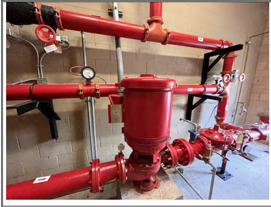
FIRE PUMP (TYPICAL)
