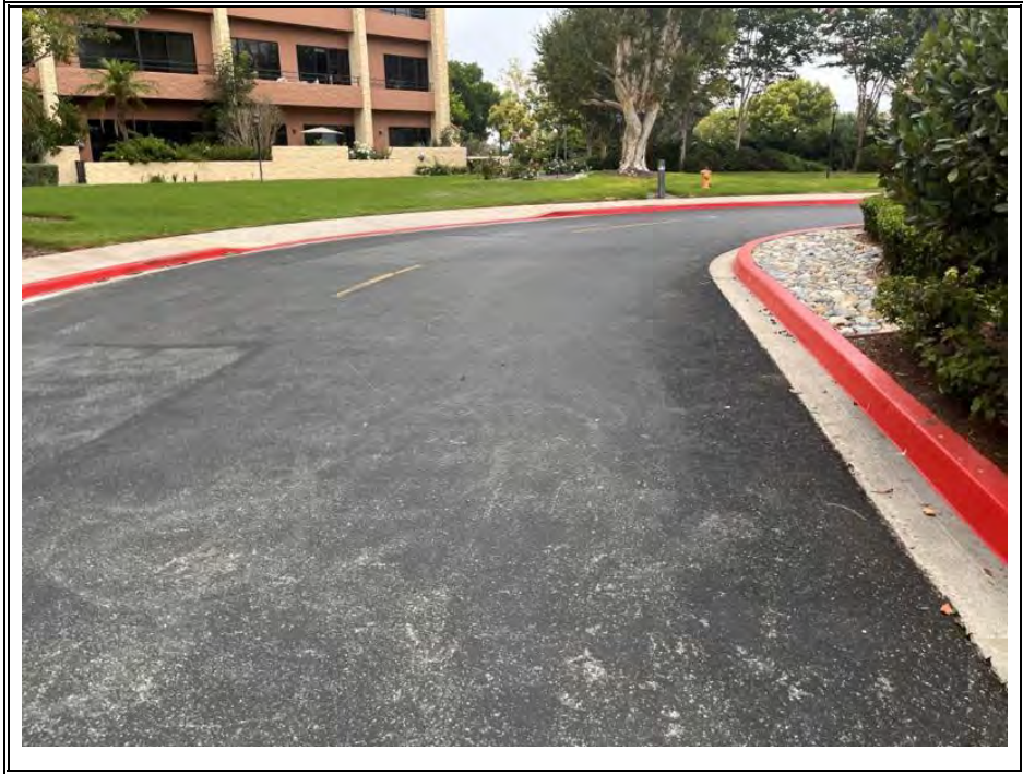
ASPHALT REPLACEMENT-NEWER (TYPICAL)
