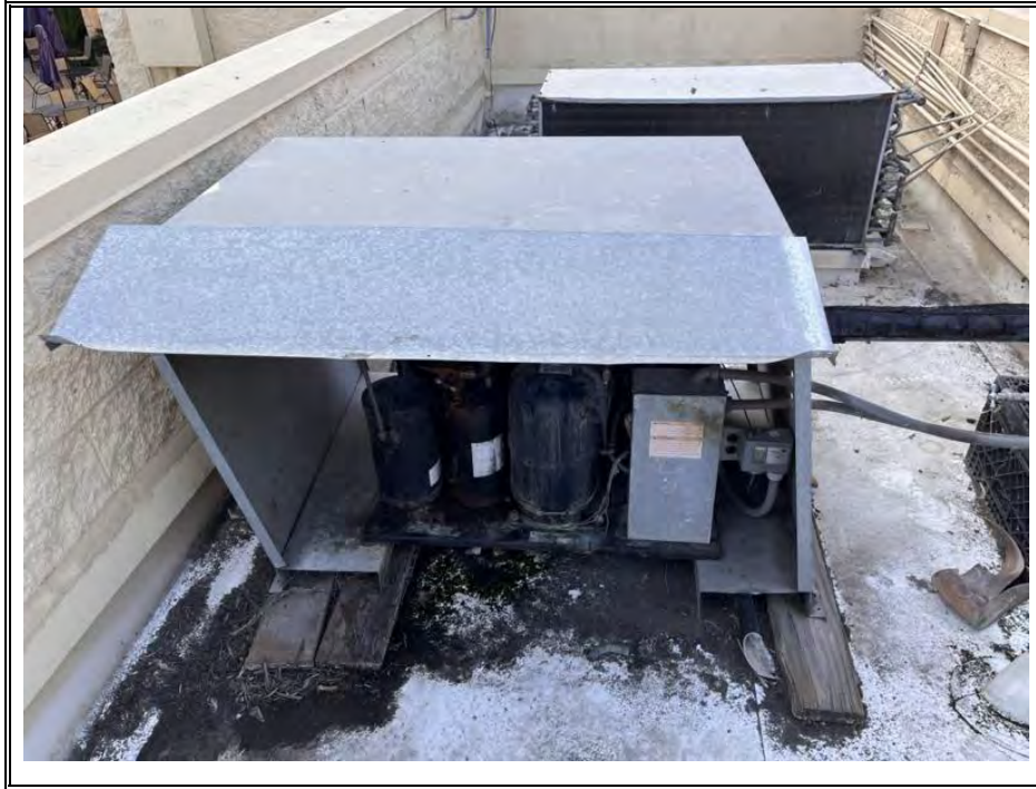
REFRIGERATION CONDENSING UNIT (TYPICAL)
