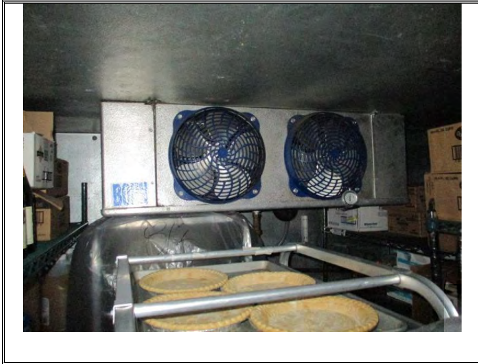
REFRIGERATION COIL-1998 (TYPICAL)
