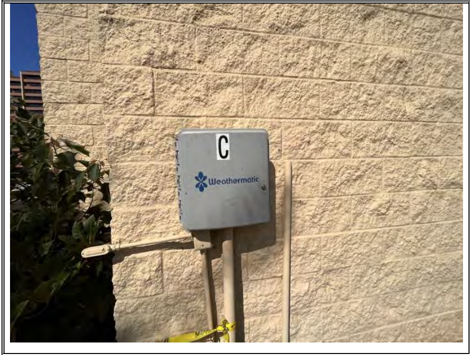
IRRIGATION EQUIPMENT (TYPICAL)
