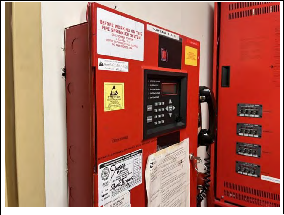
FIRE ALARM STATION (TYPICAL)
