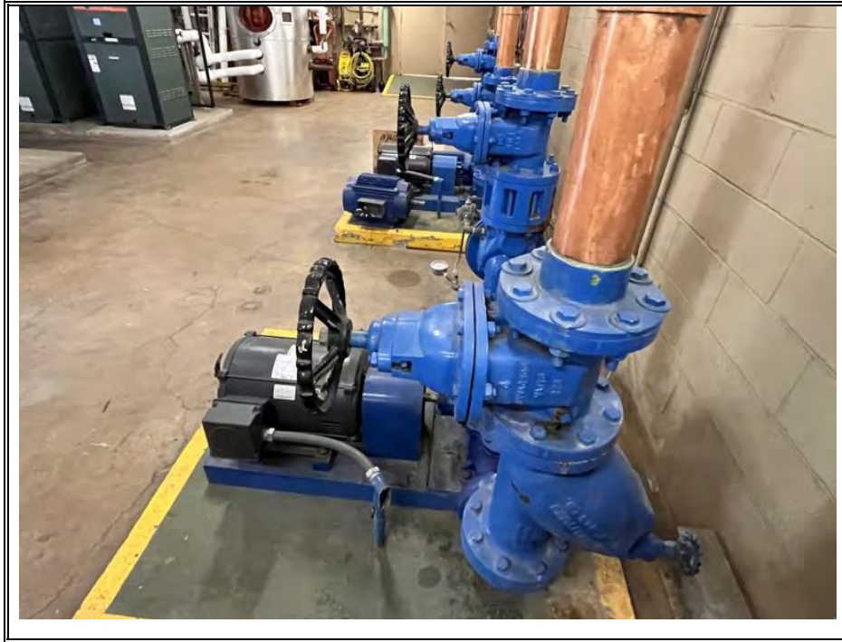
DOMESTIC WATER PUMPS (TYPICAL)
