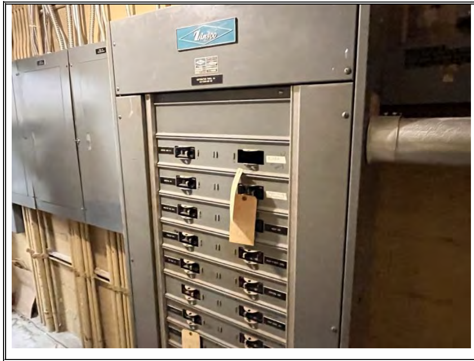
EQUIPMENT ELECTRICAL PANEL (TYPICAL)
