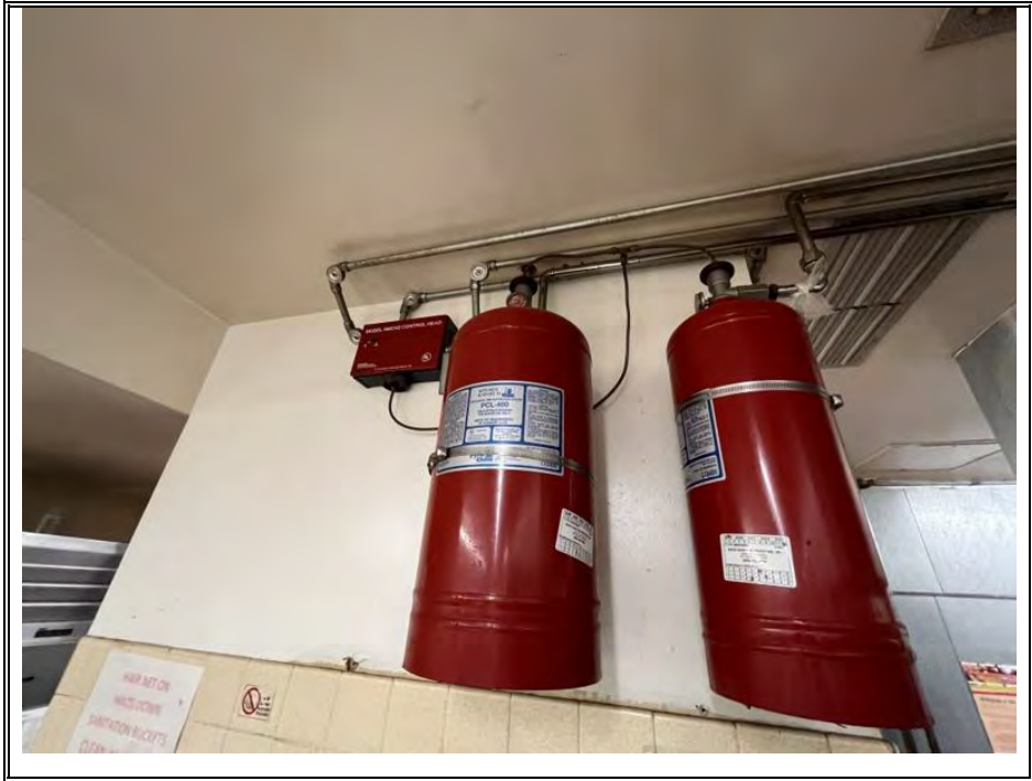
KITCHEN FIRE SUPPRESSION SYSTEM (TYPICAL)
