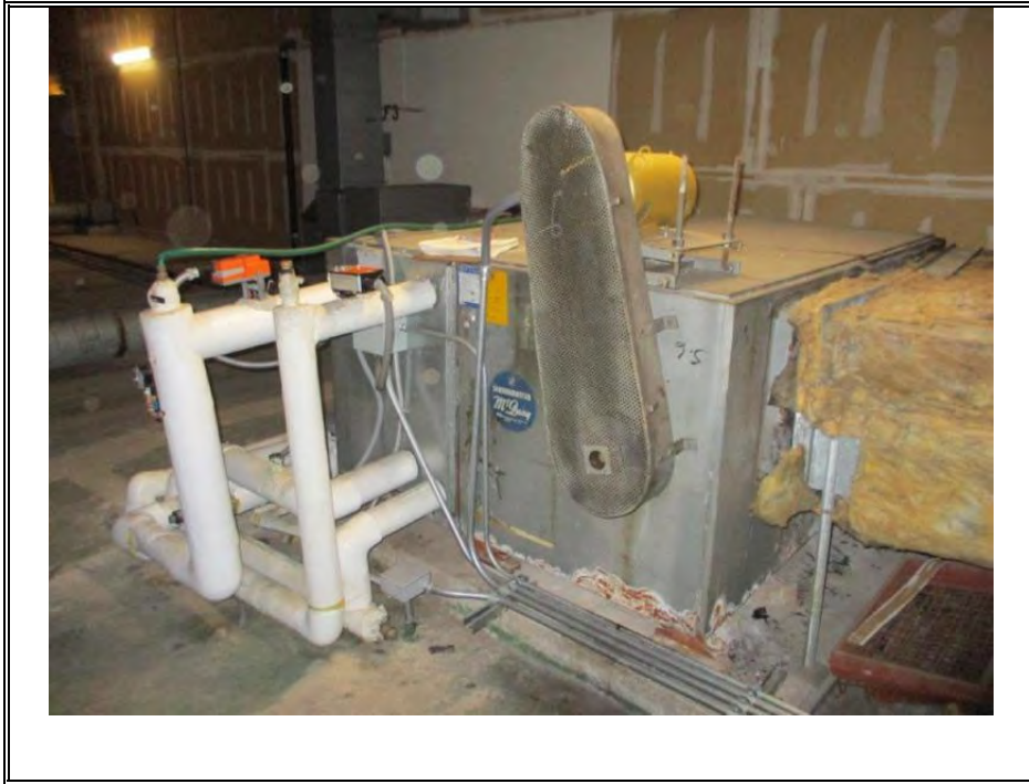
FAN COIL UNIT S-11 (TYPICAL)
