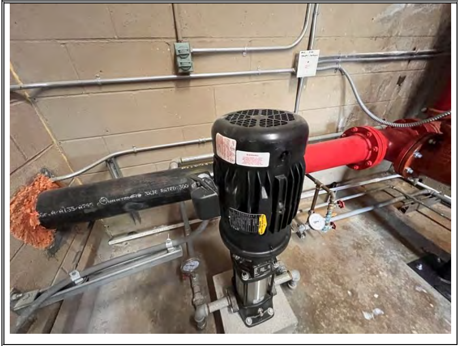
JOCKEY PUMP (TYPICAL)
