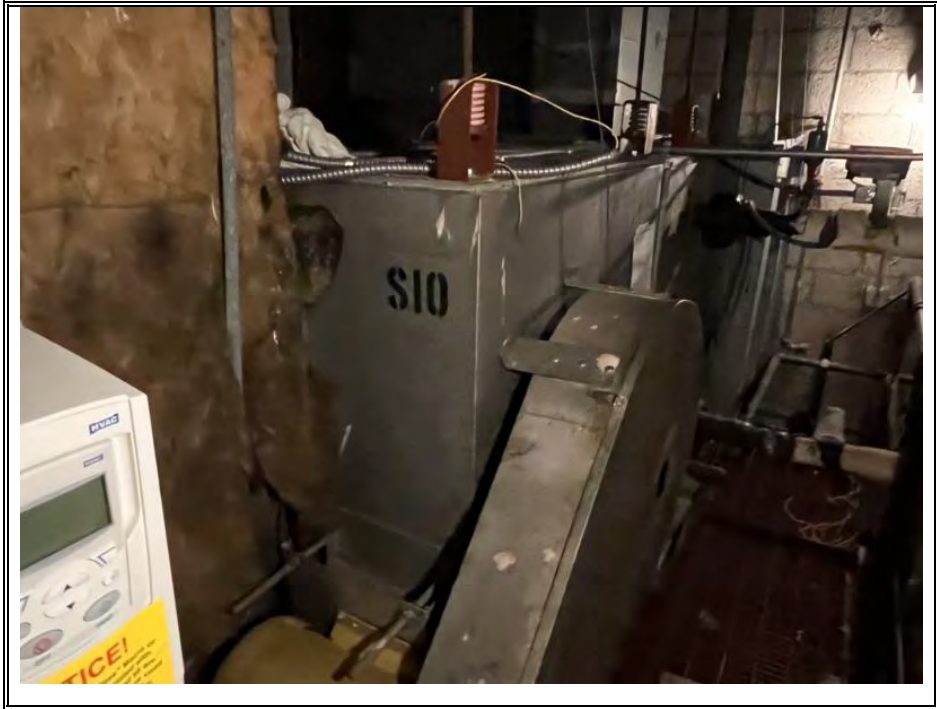
FAN COIL UNIT S-10 (TYPICAL)
