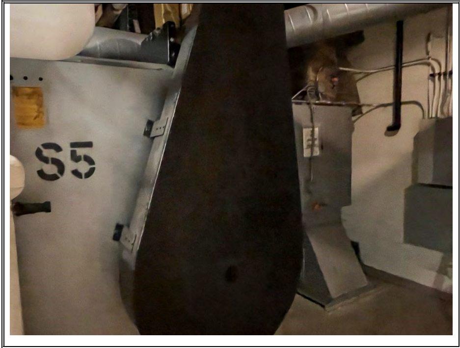
FAN COIL UNIT S-5 (TYPICAL)
