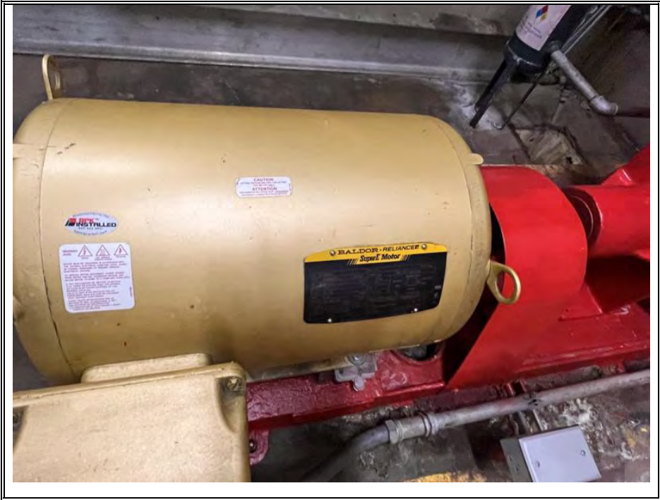
CHILLED WATER PUMPS (TYPICAL)
