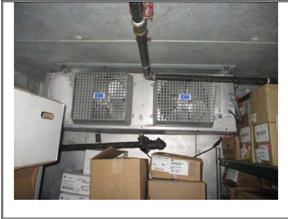
REFRIGERATION COIL-2004 (TYPICAL)
