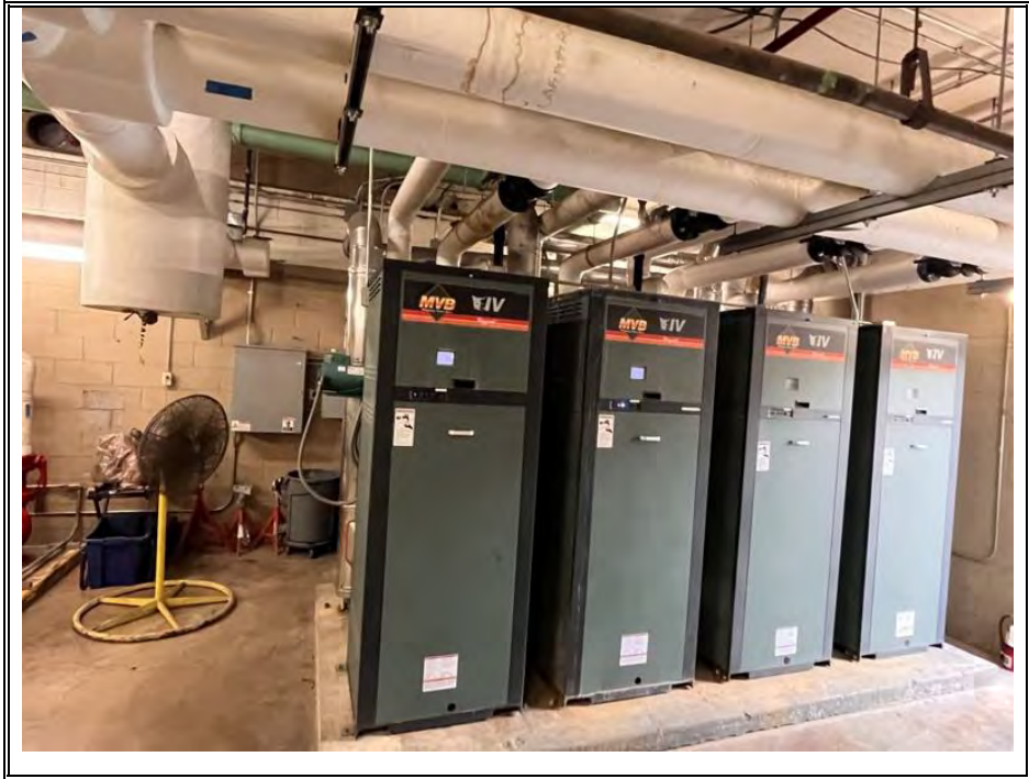
BOILERS-CLOSED LOOP SYS (2000) (TYPICAL)
