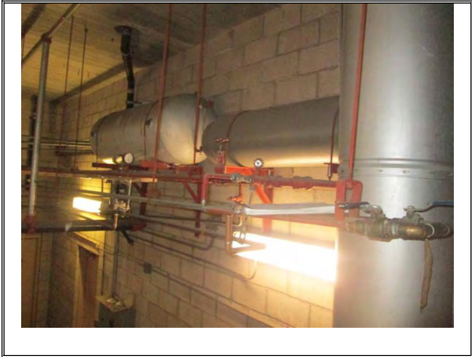
EXPANSION TANK-2002 (TYPICAL)
