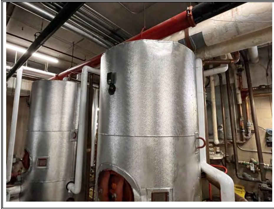
HOT WATER STORAGE TANKS (TYPICAL)
