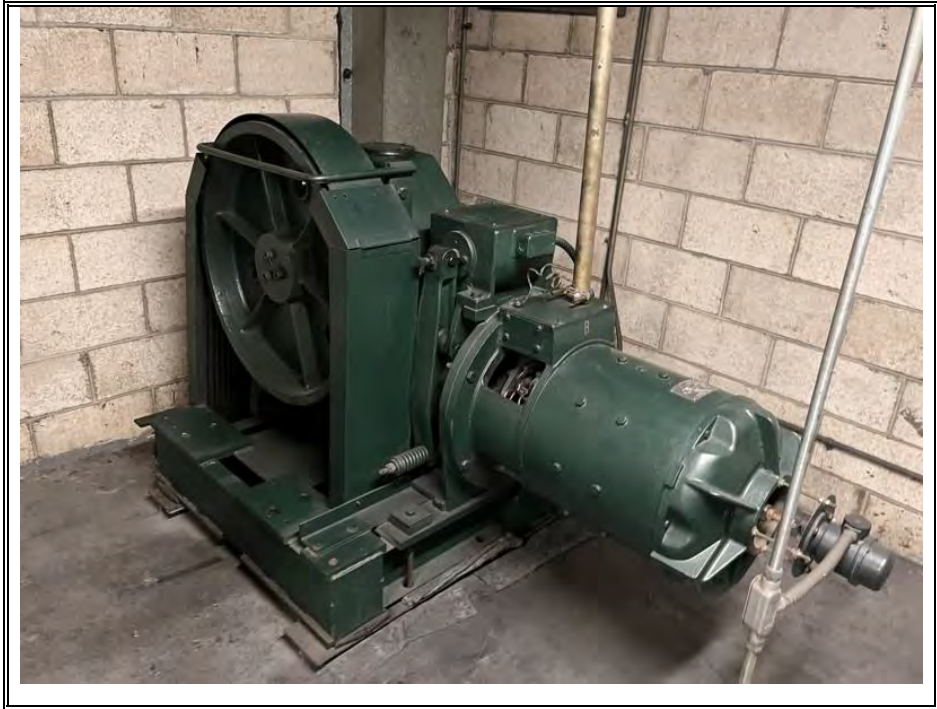
ELEVATORS-MECHANICAL (PHASE 1) (TYPICAL)
