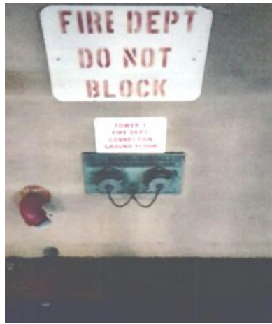
Fire Dept. Connection Tower 1 Ground Floor
