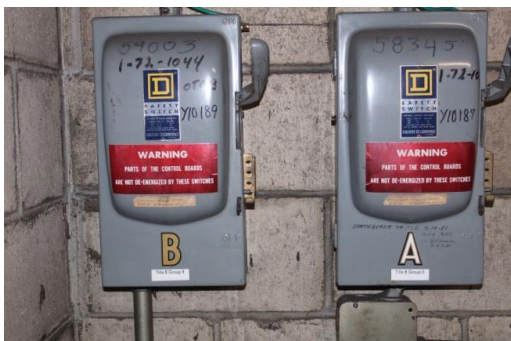
Elevator Electric Main Line Disconnect
