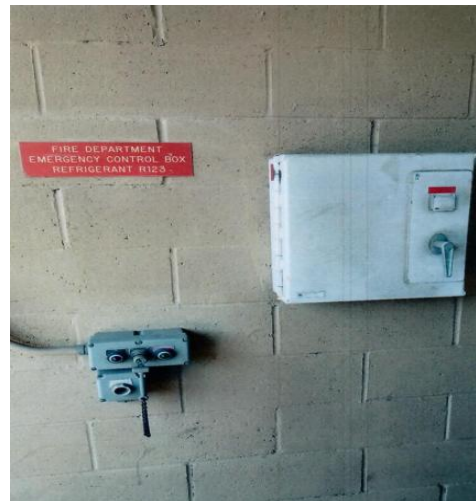
Refrigerant Emergency Control Box
