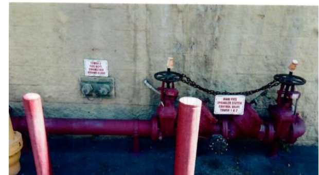
Main Fire Sprinkler System Control Valve Tower 1 & 2
