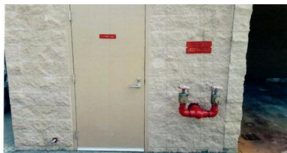
Fire Pump Room
